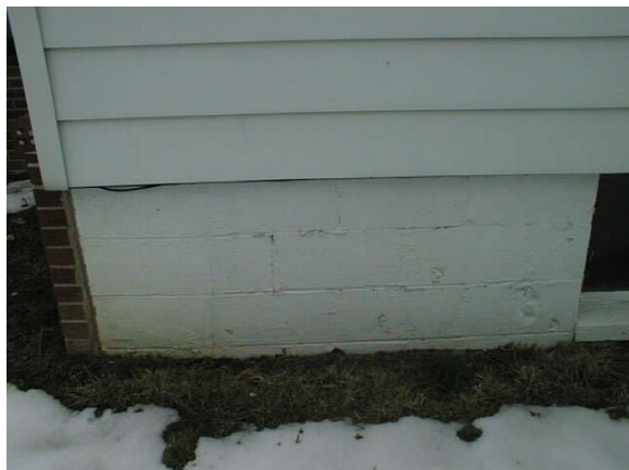
Photo 5 , Mortar joint crack in foundation, right side between corner and window.
