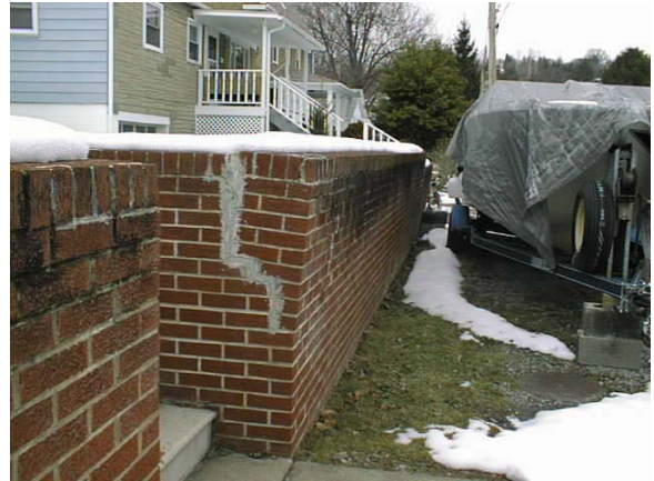
Photo 13 , Front retaining wall, leaning approximately two inches out of plumb.
