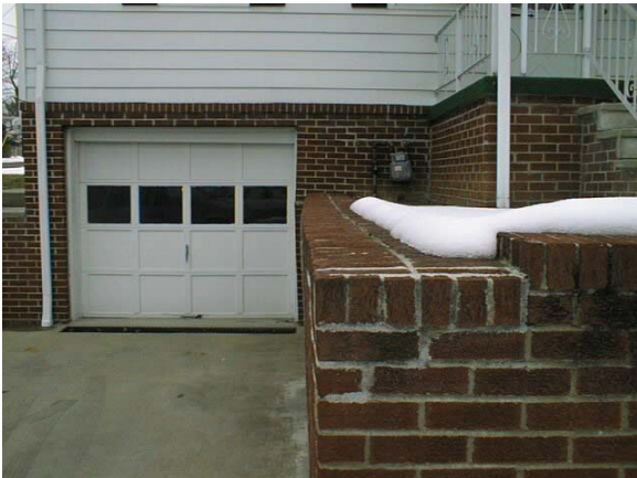
Photo 12 , Bow in driveway retaining wall.
