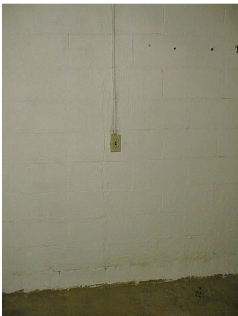
Photo 7 , Vertical hairline mortar joint crack adjacent to receptacle on front wall, near corner.
