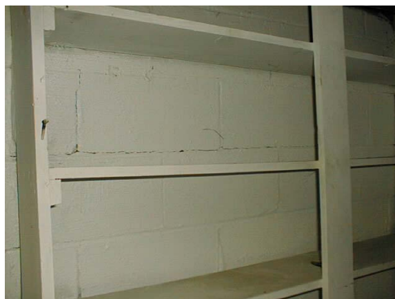
Photo 9 , Horizontal mortar joint crack on rear wall between pilasters.
