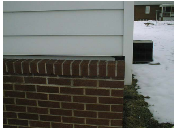
Photo 4 , Brick settled between porch and corner. Note exposed wood header board.
