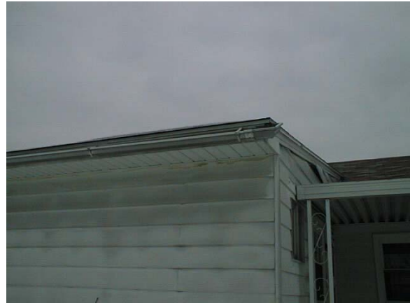
Photo 2 , Gutter on rear of addition coming loose. Siding loose over roof as well.
