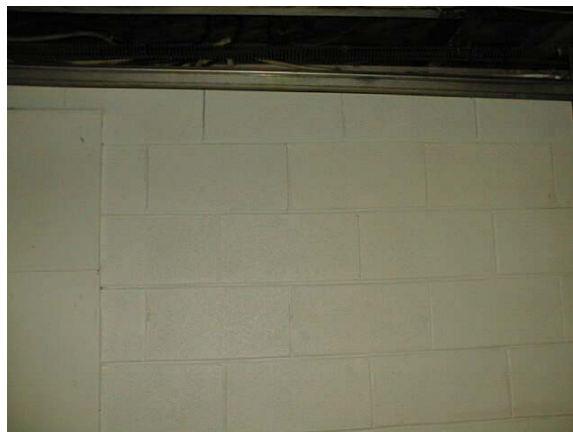
Photo 8 , Mortar joint crack to the right of the electric panel, left wall.
