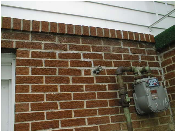
Photo 3 , Mortar joint cracking in brick behind gas meter.
