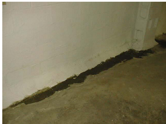
Photo 16 , Showing water exiting the wall at the bottom of the B-bond.
