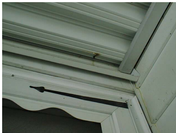
Photo 11 , Leak in rear awning above door.
