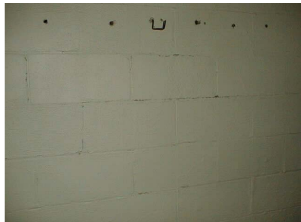
Photo 6 , Stair-step mortar joint crack on front wall in basement.
