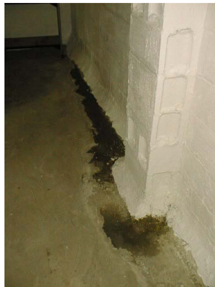
Photo 15 , Water along right foundation wall, taken 2-12-00.
